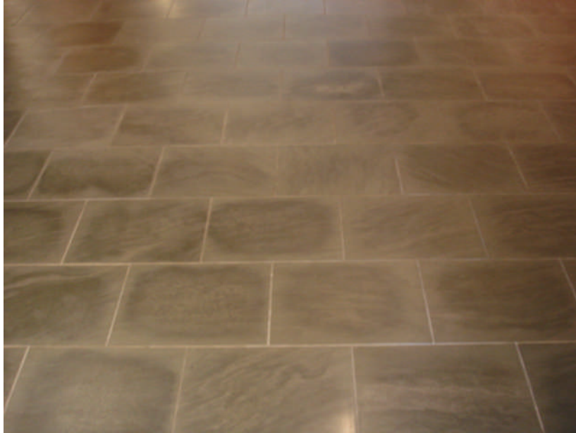
Figure 3 – discoloration of honed Pietro di Cardoza sandstone caused by prolonged exposure to residual adhesive moisture after installation over an impermeable crack-isolation membrane; note the “halo” at the perimeter where moisture escapes through grout joints
