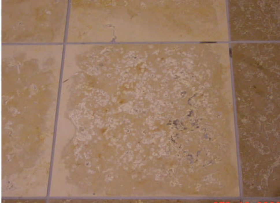
Figure 2 – honed limestone tile with reactive organic content damaged from excessive moisture exposure resulting from failure to install vapor retarder
